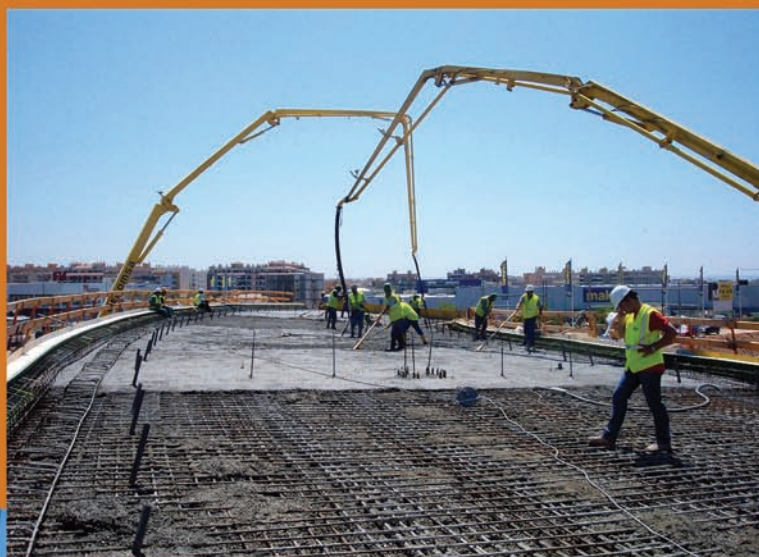
Bridge between the industrial parks in Palma de Mallorca. Opened in July 2005.
