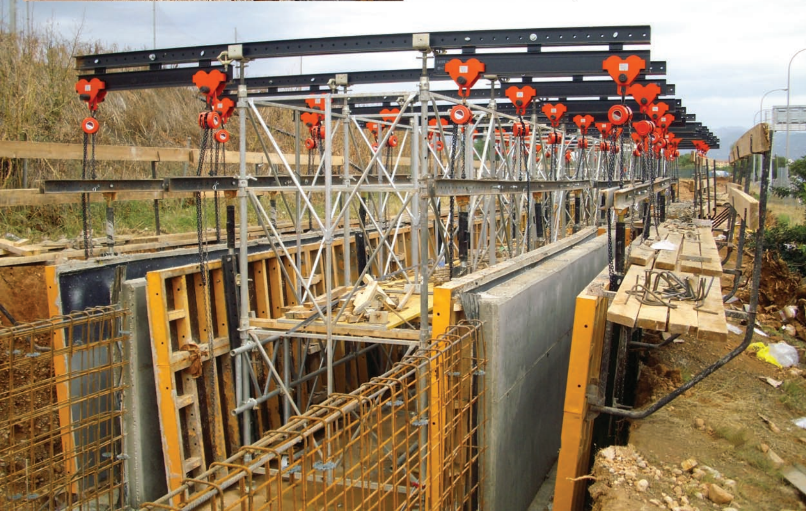
Works of water collector of Palma subway.
